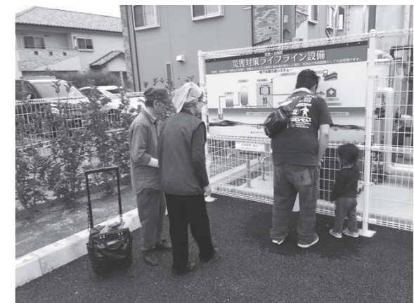
Groundwater membrane filtration system installed at a hospital in Kumamoto City. Water was provided to nearby residents during the Kumamoto earthquake.
